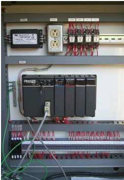
PLC (Programmable Logic Control)
